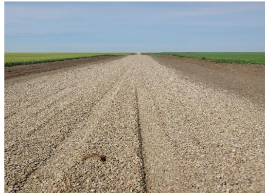
Figure 8. Rng Rd 18-3 South of Twp Rd 6-0
